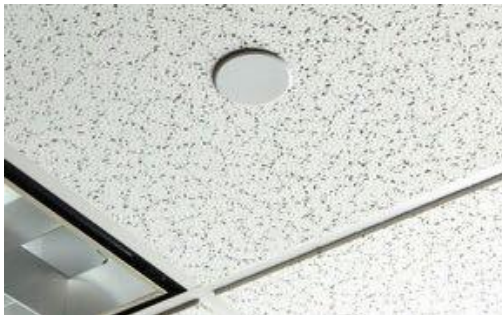
Concealed fire sprinkler heads with cover plates
