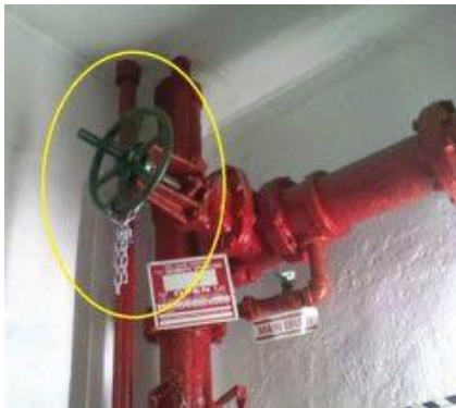
The green valve is a floor control valve. In this photo, the control valve is in the open position.
