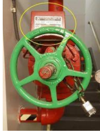
Tamper switch on a sprinkler valve
